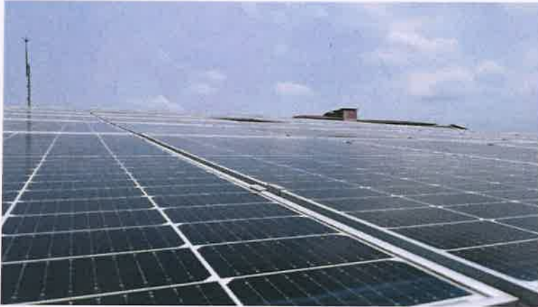
Figure 8 25 kWp SOLAR POWER PLANT
