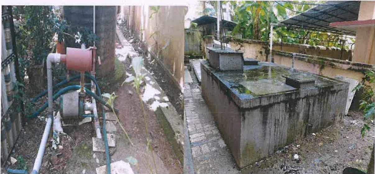
Figure 13 BOREWELL AND WATER TANK
