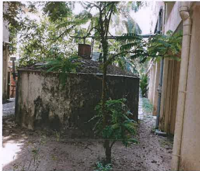
Figure 14 RAIN WATER COLLECTION TANK
